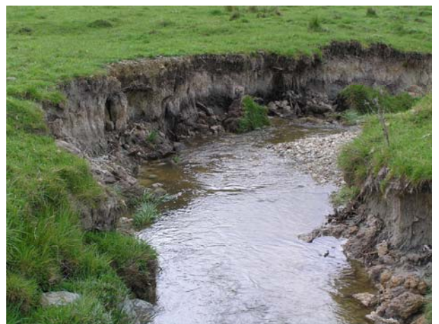
Slab failures and bank undercutting, Motueka River
