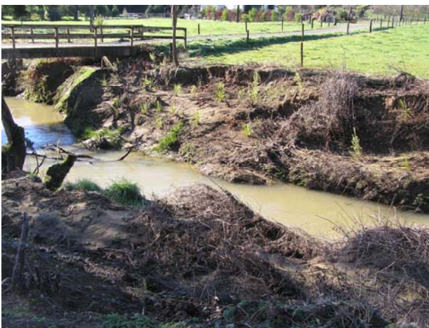
Slump failures, Raglan
